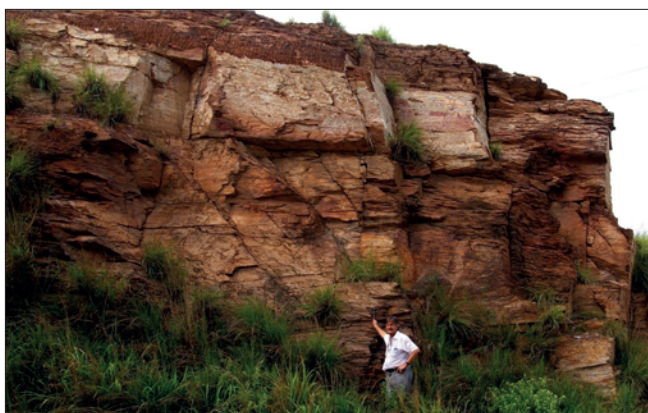
Fig. 8. Precambrian age granitic gneiss in the interior of Angola. Note the vertical and oblique orientation of the fractures which indicates this would be a complicated potential oil-producing reservoir. Note also that it is not intensely fractured like the granite in Fig. 7. Accordingly, this reservoir would be inferior in comparison to the reservoir which outcrops in Fig. 7 (Koning, 2014).
