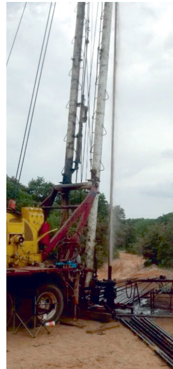
Fig. 2. Picture of mixture gush (water – 70%, oil – 30%) from the well No.8.
