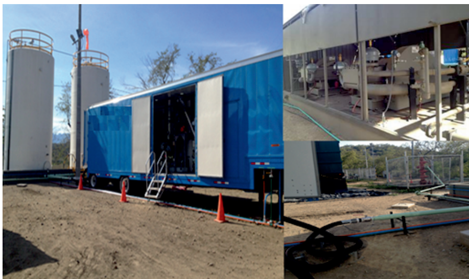
Figure 11. Polymer flooding pilot facilities in the injection wells.
